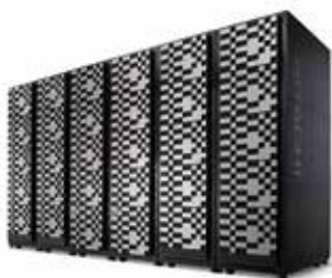
A storage system
